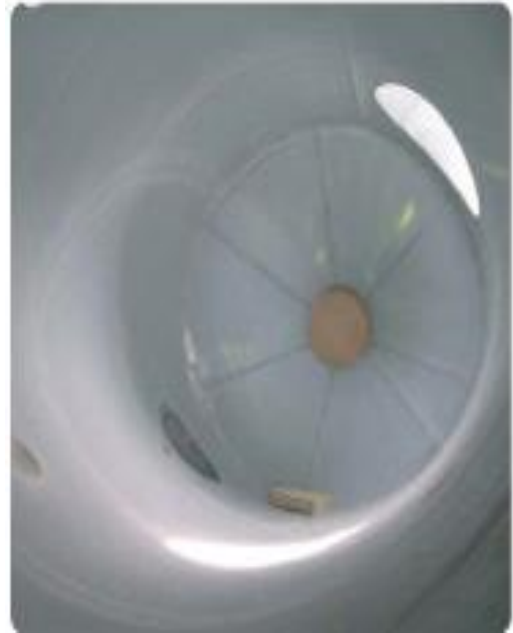
PVDF Tank Lining
